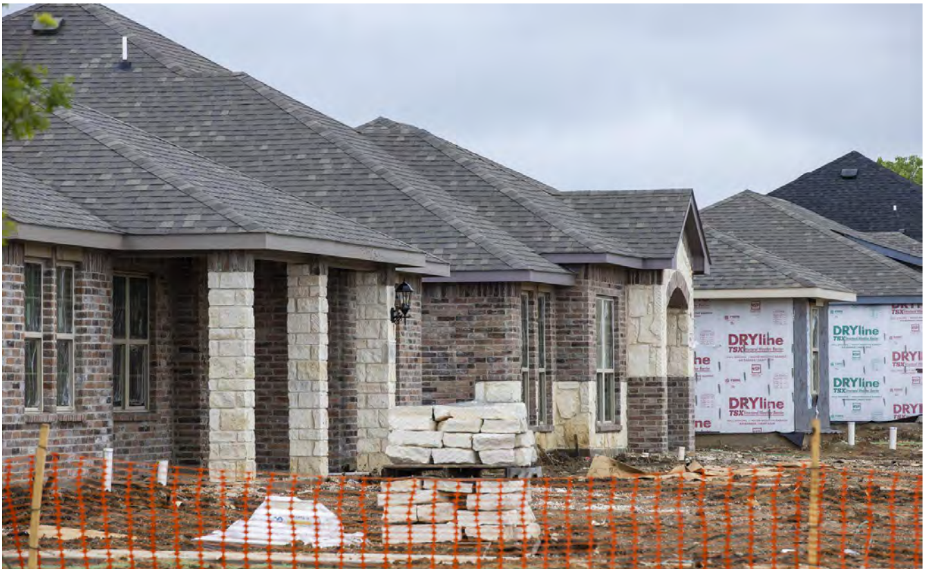
Construction was underway last month on houses in Kensington Valley by Camden Homes in southeast Dallas. The community is near the intersection of Interstates 635 and 20 and has 112 homes. (Lynda M. González / Staff Photographer)
